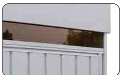
Front Skylight Window for Natural Daylight
