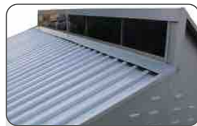
Front skylight window for natural daylight
