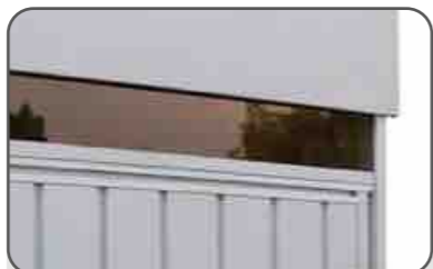
Front Skylight Window for Natural Daylight
